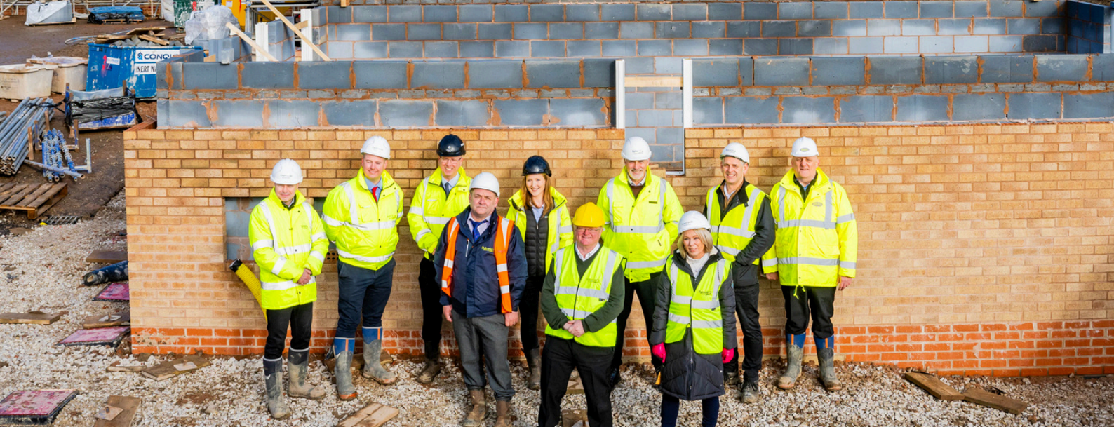
70 new homes are being built on the Whiteleas Avenue site at North Wingfield Progress visit to site included Rykneld Homes staff, Countryside Partnership staff and Cllr Nigel Barker
